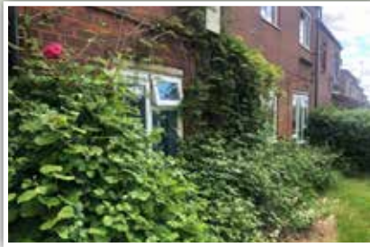
Photo showing the encroachment before the work
